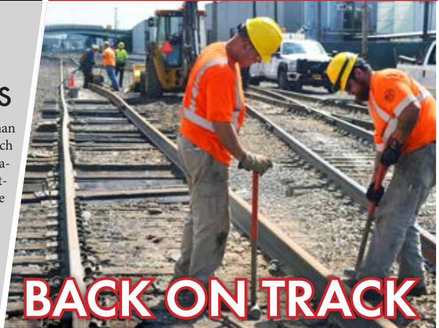
Welder Helper Andrew Clark, left, works with Sectionman Jeremiah Mettler on Portland Terminal tracks.
