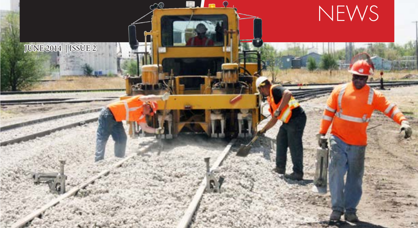
Wichita Terminal Association employees raise the track above ground level. From left are Laborer Matt Jacobs, Track Supervisor/Tamper Operator Jason Smith, Section Foreman Royce Franklin and Truck Driver/Laborer Terry Shine.
